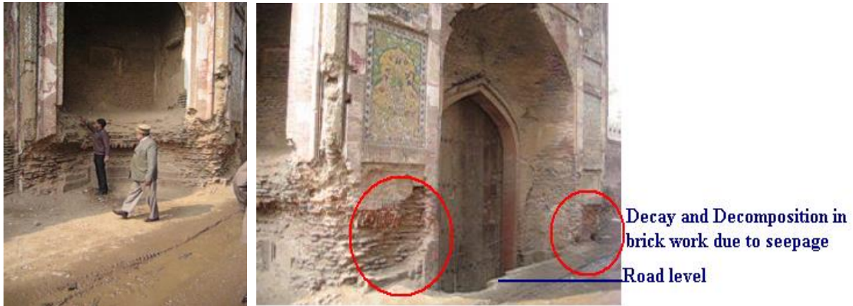
Figure – 10: Picture showing the northern main gate of Shalimar Garden. The levels of the surrounding road is higher than the natural ground level of the garden, causing water ingress in the foundations.
