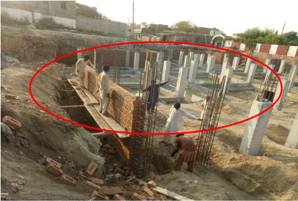
Figure No 3: Personal protective equipment's not available at site
