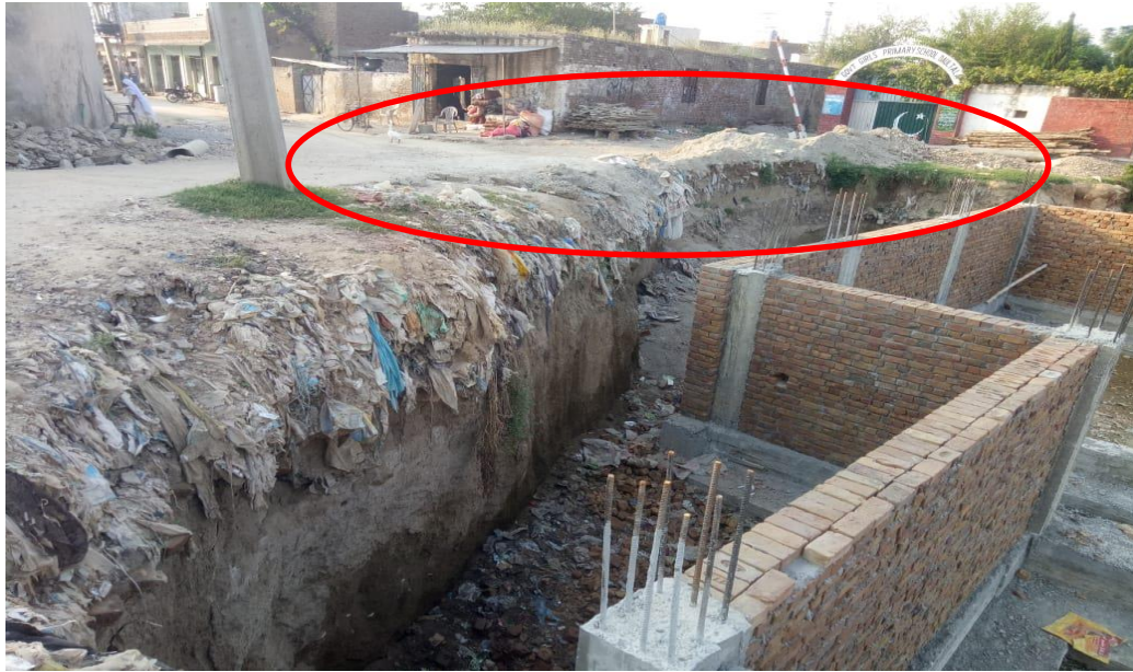
Figure No 5: No boudary wall and warning signs
