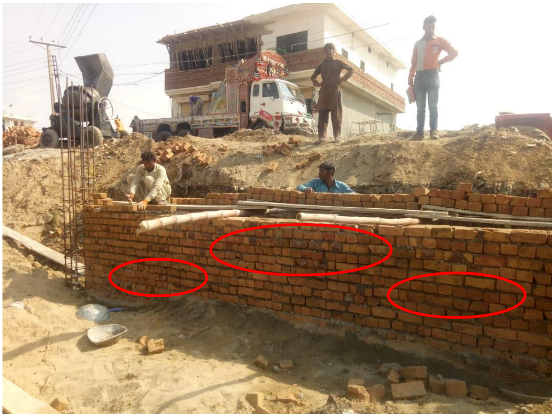
Figure No 8: Broken bricks and second class over burned bricks
