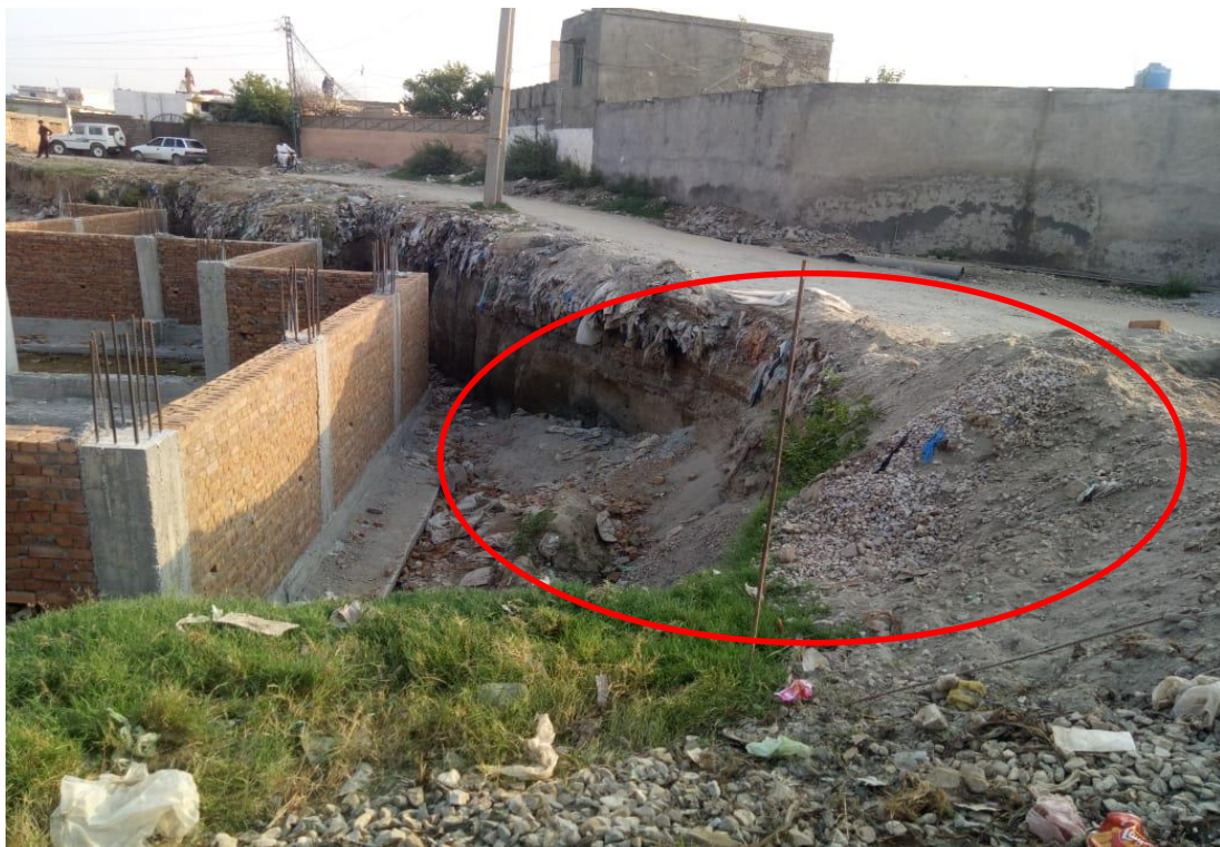
Figure No 6: No warning signs and safety belt
