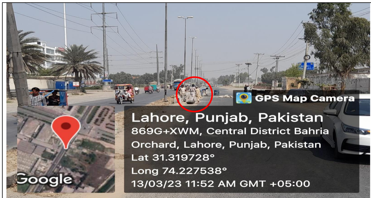
Fig No. 3: Labor was not provided with Personal Protection Equipment
