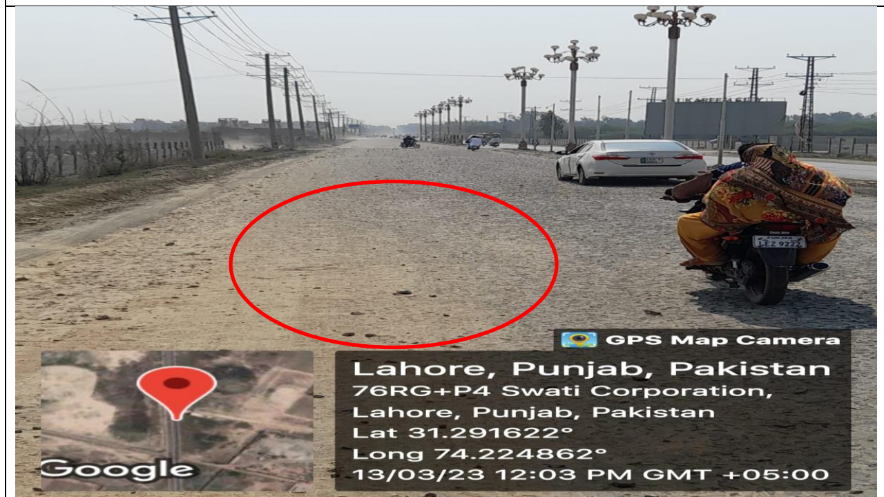
Fig No. 2: Water bound particles were disintegrated from the surface due to poor compaction
