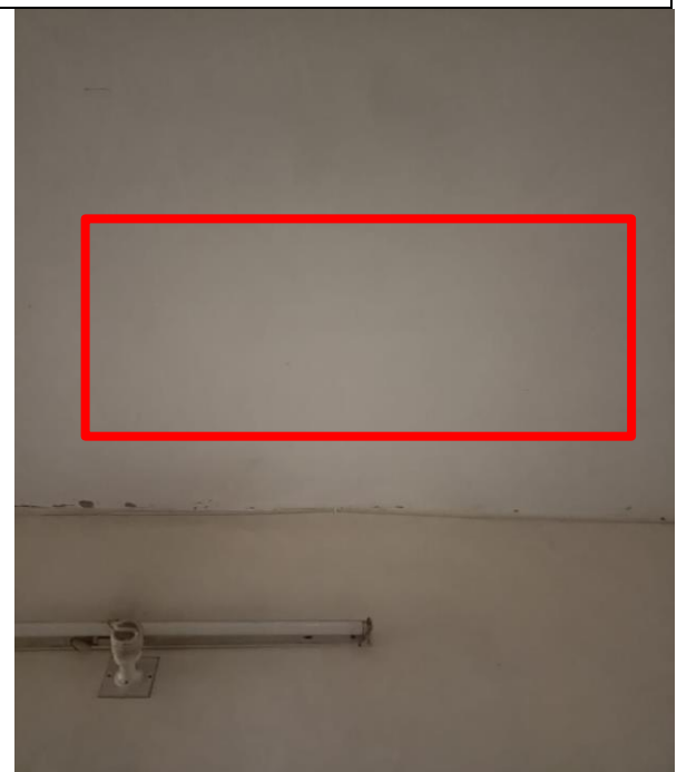
Figure 12: Cracks propagating towards roof slab was partially retified
