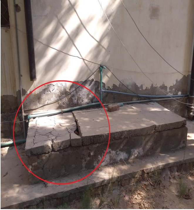
Figure 25: Broken slab of sanitary chamber
