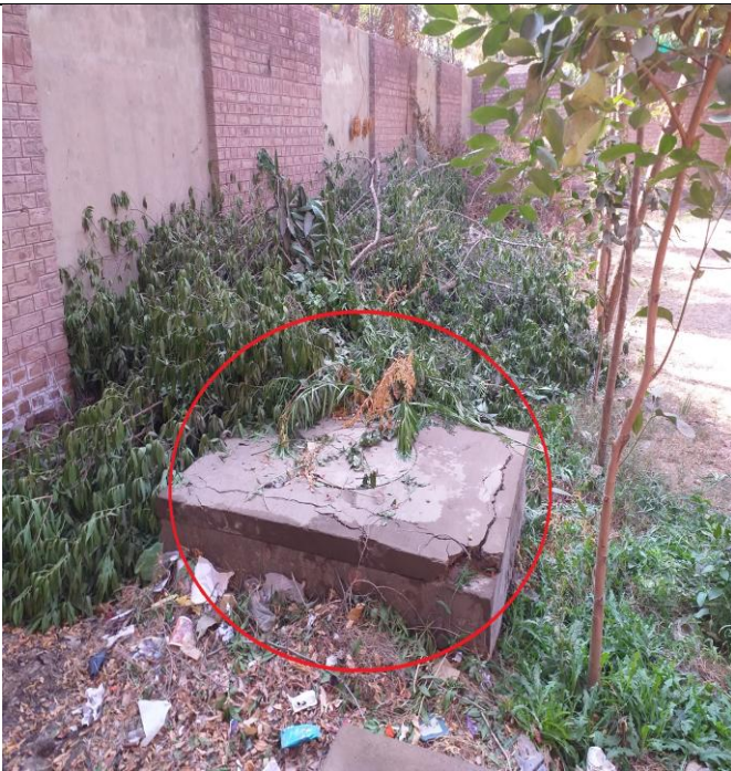
Figure 27: Broken slab of man-hole
