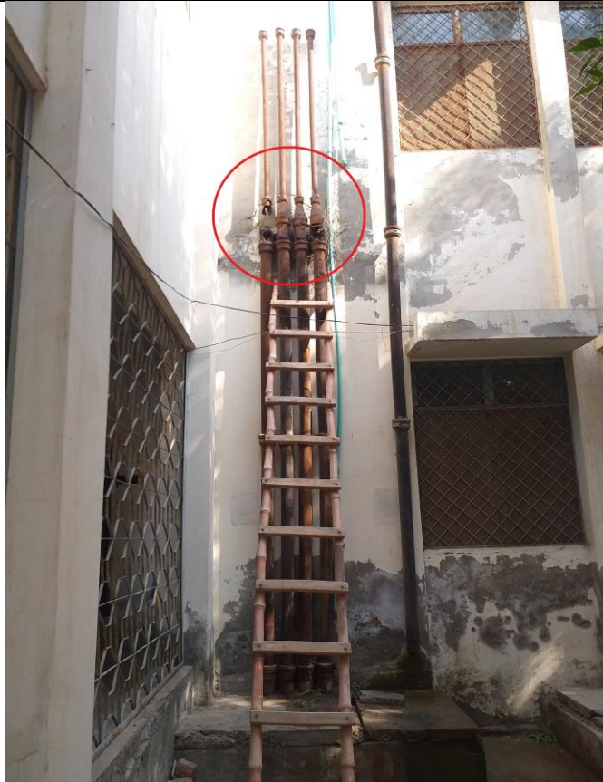
Figure 29: Broken and rusted sewer gas smell vent pipe
