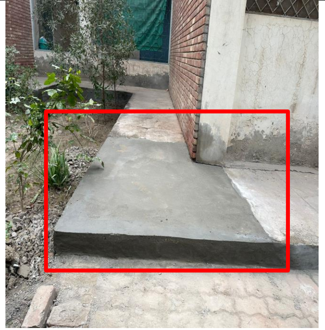
Figure 22: Broken outer protection flooring was rectified
