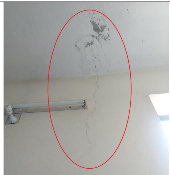
Figure 11: Cracks propagating towards roof slab
