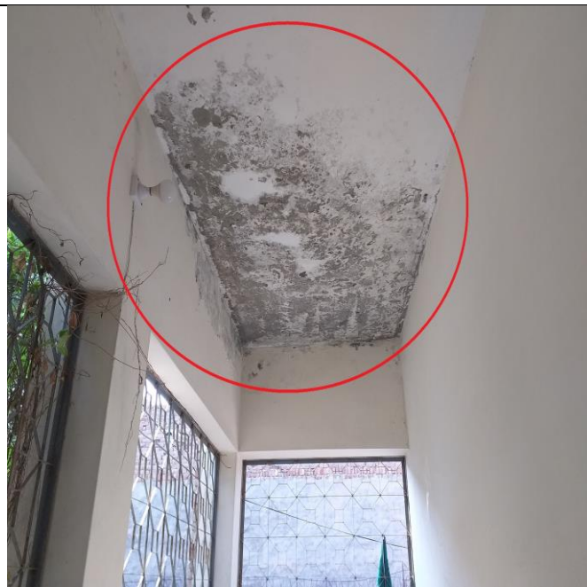
Figure 7: Issue of seepage and dampness in the roof slab of the building
