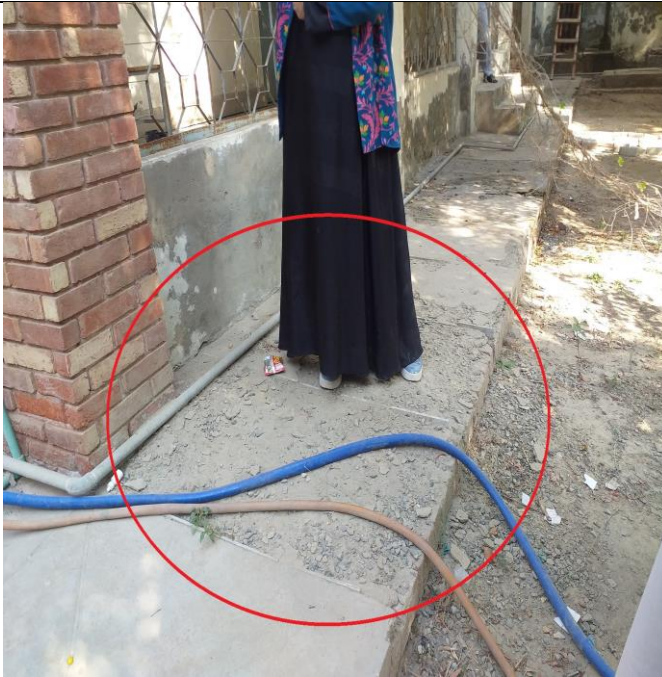
Figure 23: Damaged PCC of flooring
