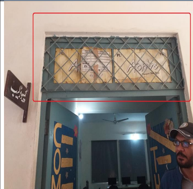
Figure 9: Glass of transom was broken
