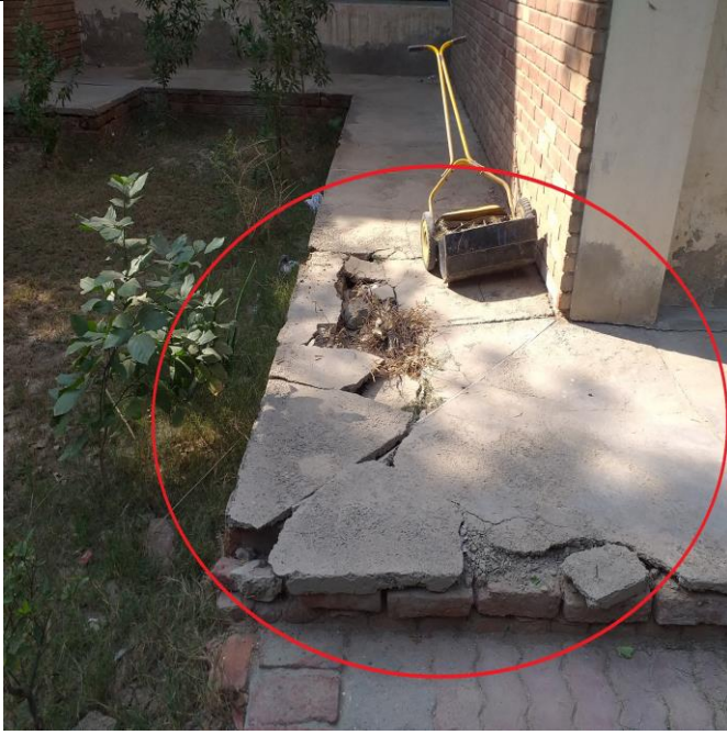
Figure 21: Broken outer protection flooring
