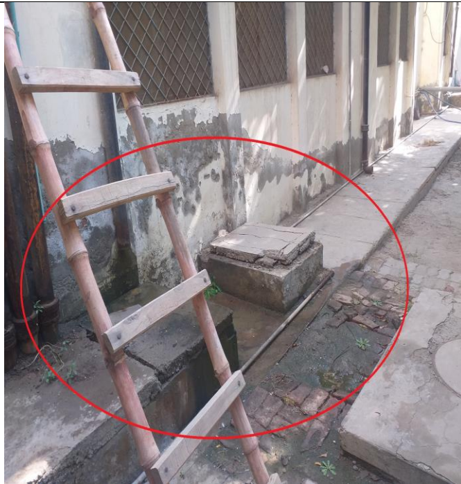
Figure 31: Seepage and infiltration due to broken pipes
