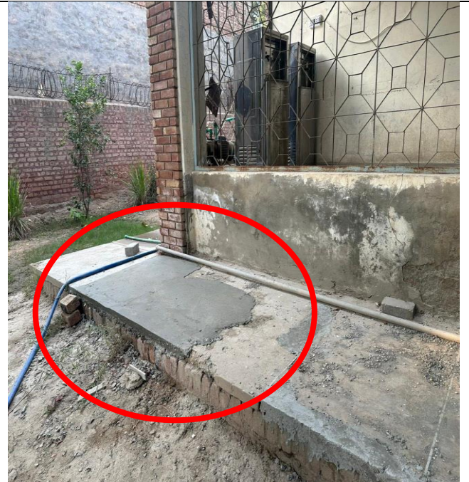
Figure 24: Damaged PCC of flooring was rectified
