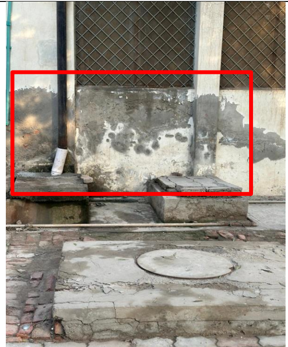
Figure 32: Seepage and infiltration due to broken pipes was partially rectified
