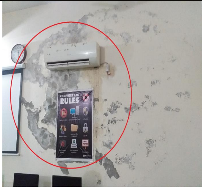
Figure 5: Issue of seepage and dampness in the walls of the building
